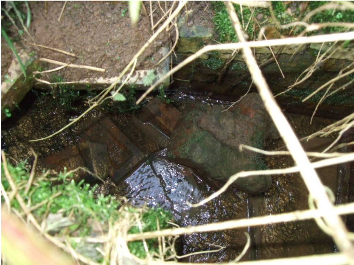
Photograph 20 Collapsed brick culvert in central part of site
